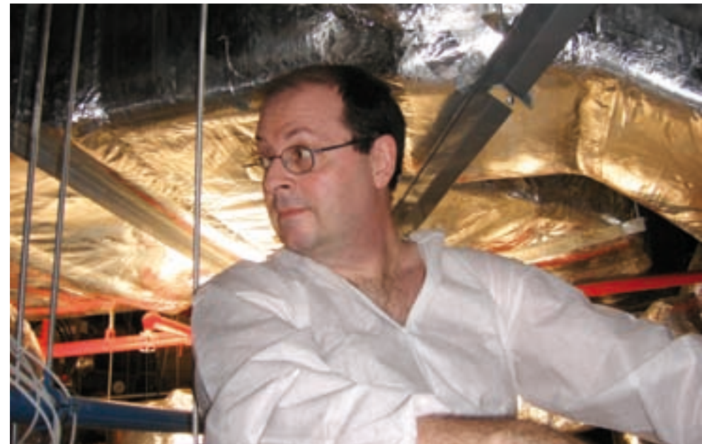
Dr. Charles Taillens casts an eye over the BSL3 air-conditioning system
